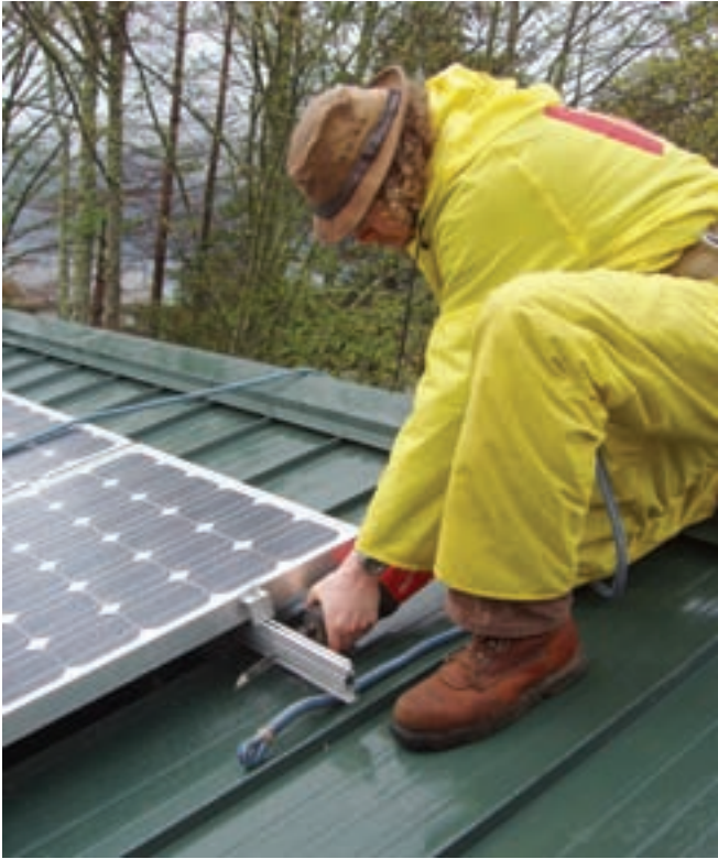
Excess length is trimmed off the array rack's rails for a neat, streamlined installation.
