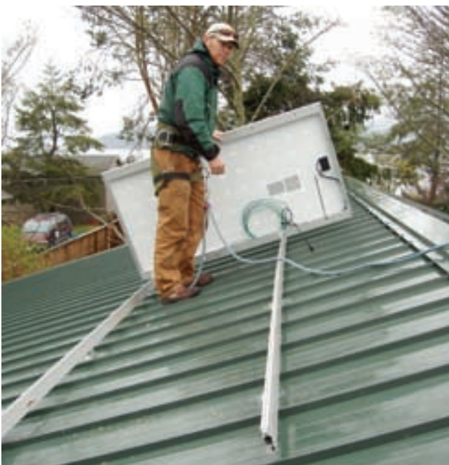
A rack mounted to the metal roof supports the photovoltaic modules.
