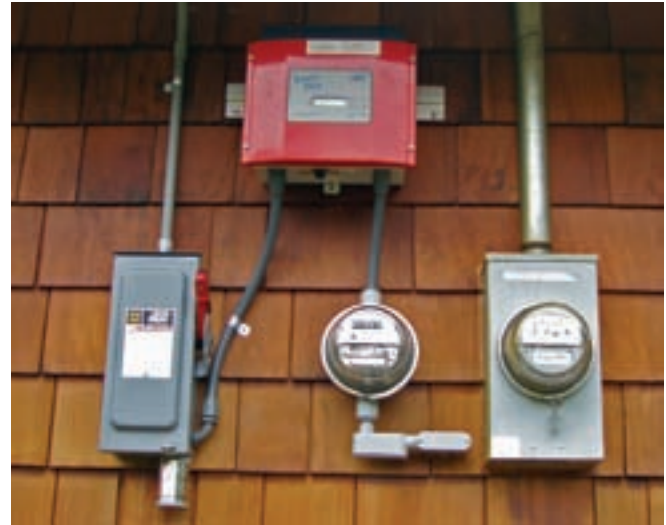
A batteryless grid-tie system is relatively simple—all components, except for the solar-electric array, are pictured here.
