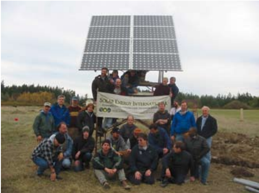
Proud PV installation workshop group after connecting the Anderson's Store PV array to the power system and the grid.
