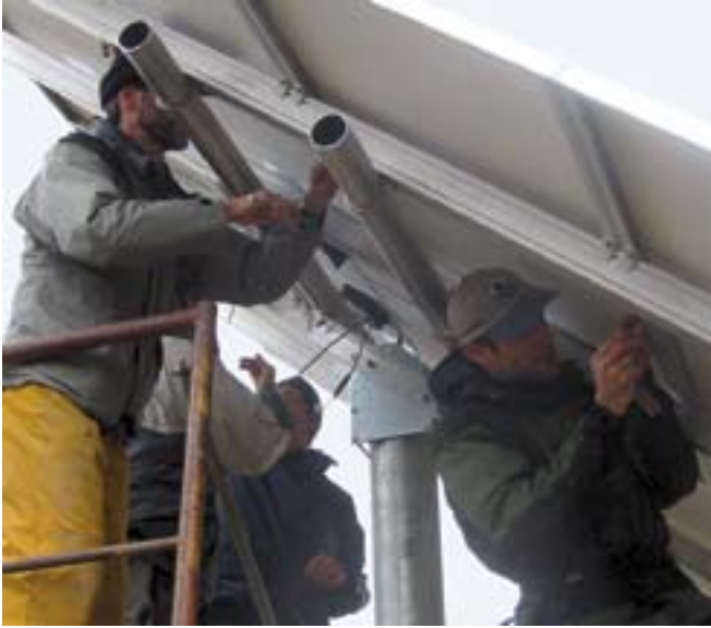
SEI students Larry Owens (left) and Tom Brenton fastening PV modules to the top-of-pole rack.
