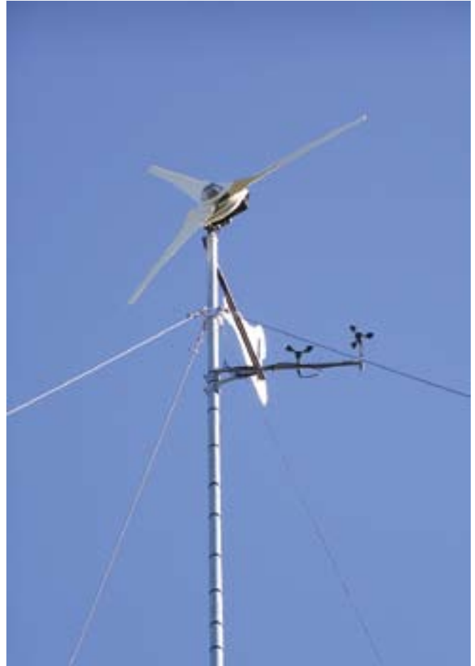
Fully installed turbine. The two anemometers supply wind data, which is accessible at the tower base and inside the power room.
