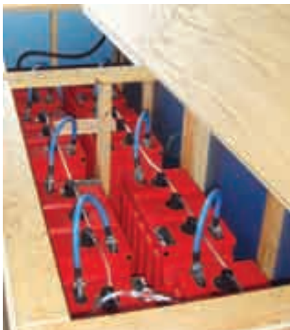
Large battery banks and engine-generators are commonplace components in off-grid systems, and significantly increase the initial and long-term operating costs.
