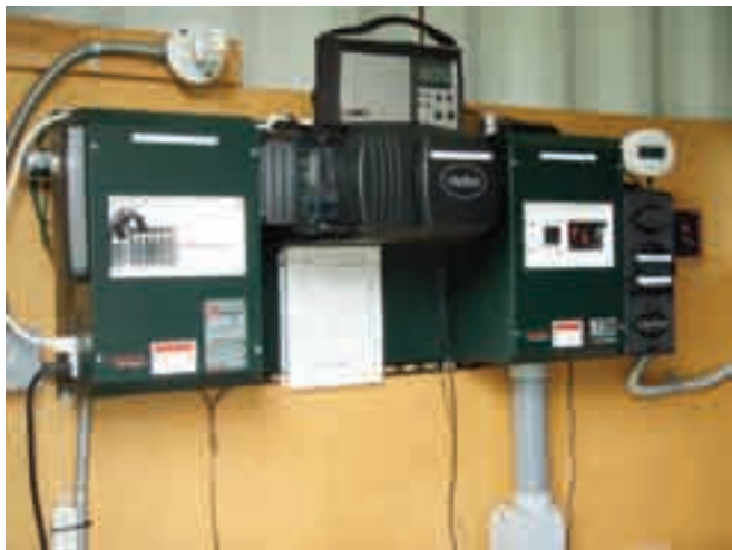
An off-grid system will require batteries and a charge controller, as well as an inverter and disconnects common to all system configurations.
