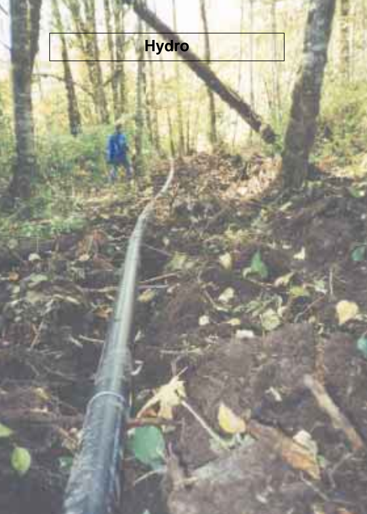
The penstock, still propped over the ditch for ease of gluing, snakes its way down to the turbine.
