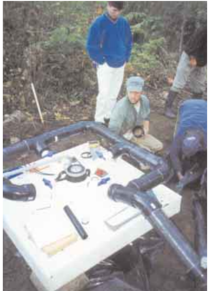
The completed manifold with the ES&D turbine.
