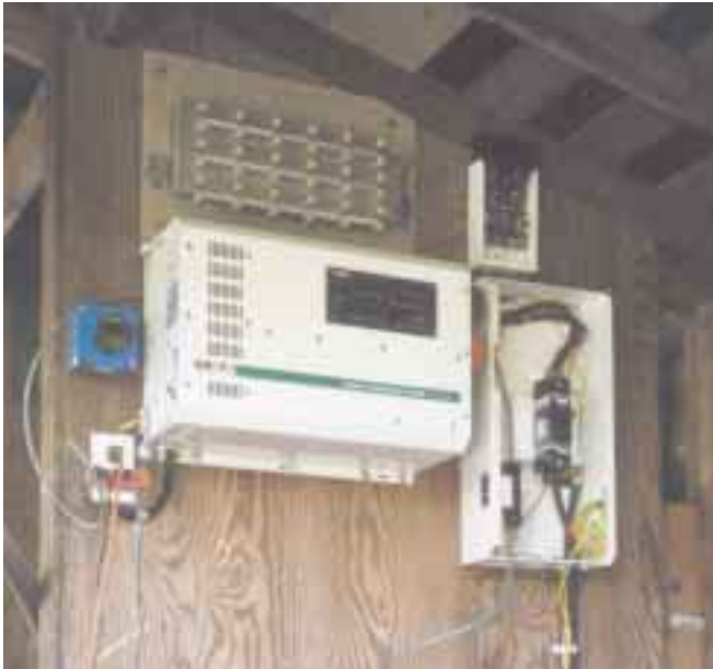
The inside of the power shed, showing inverter, DC disconnect box, charge controller, and dump load.
