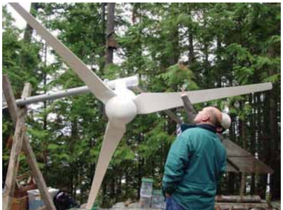
The complete AWP wind turbine was bolted to the tower’s top section prior to lift.
