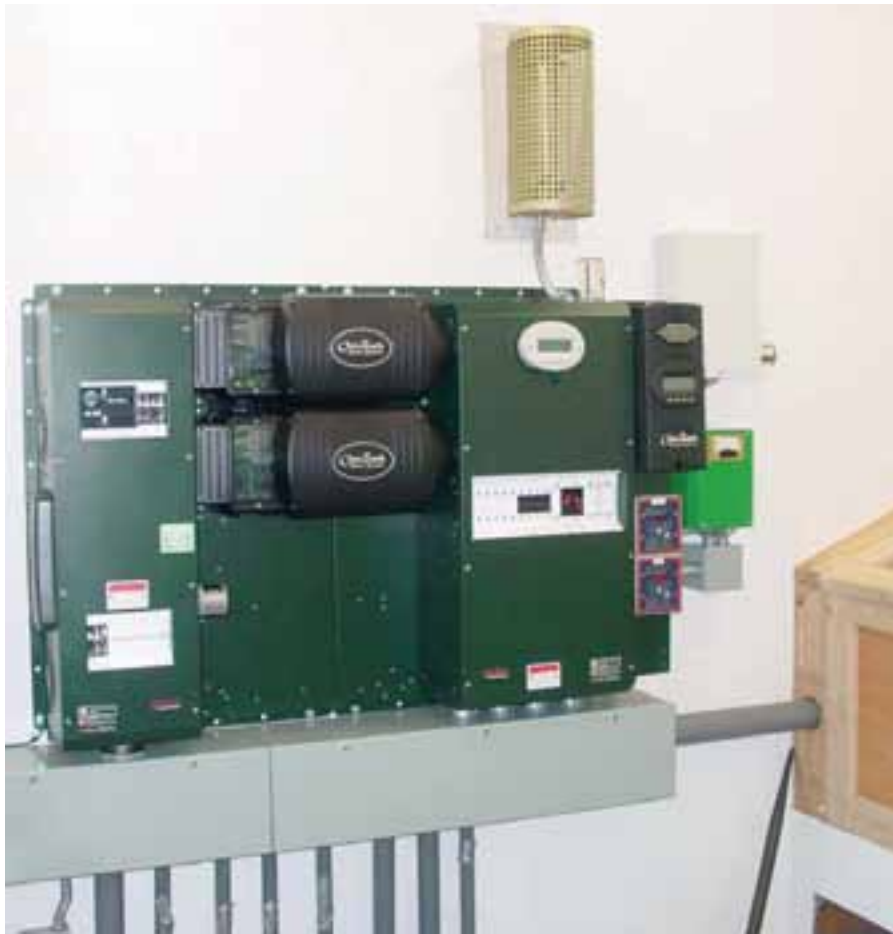
An OutBack charge controller and inverters are housed in the power shed, which is also home to a dump load, weather monitoring equipment, and the battery bank.
