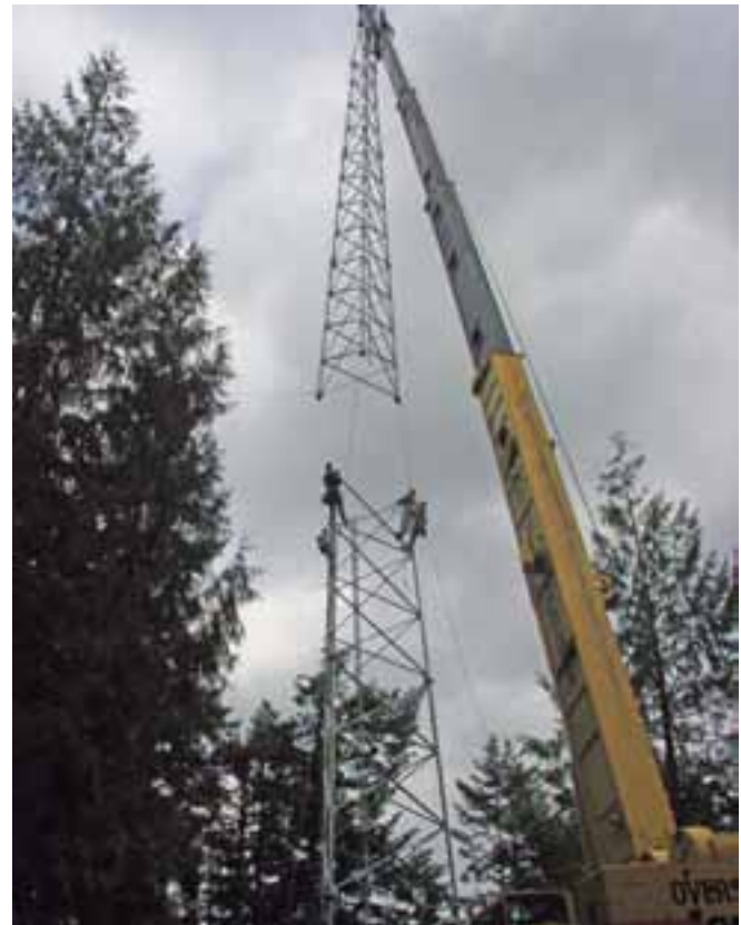
The crew at the top of the tower's first section gets ready to receive and bolt the second section into place.
