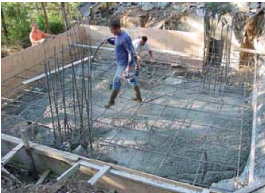
Reinforcing steel and bolts were set into the foundation before pouring concrete.
