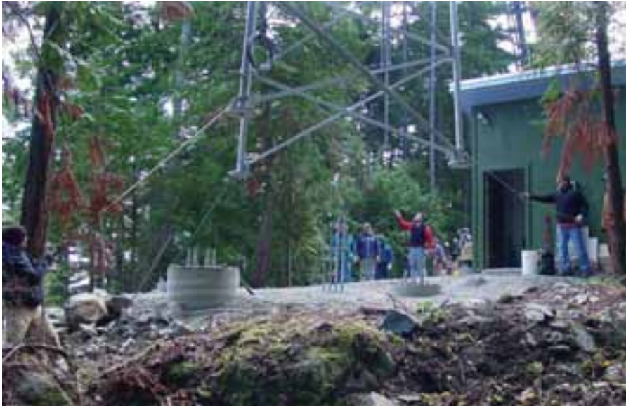
A 50-ton crane lifted each assembled tower section into place. Amazingly enough, the first section lined up perfectly with the column bolts set into the concrete.
