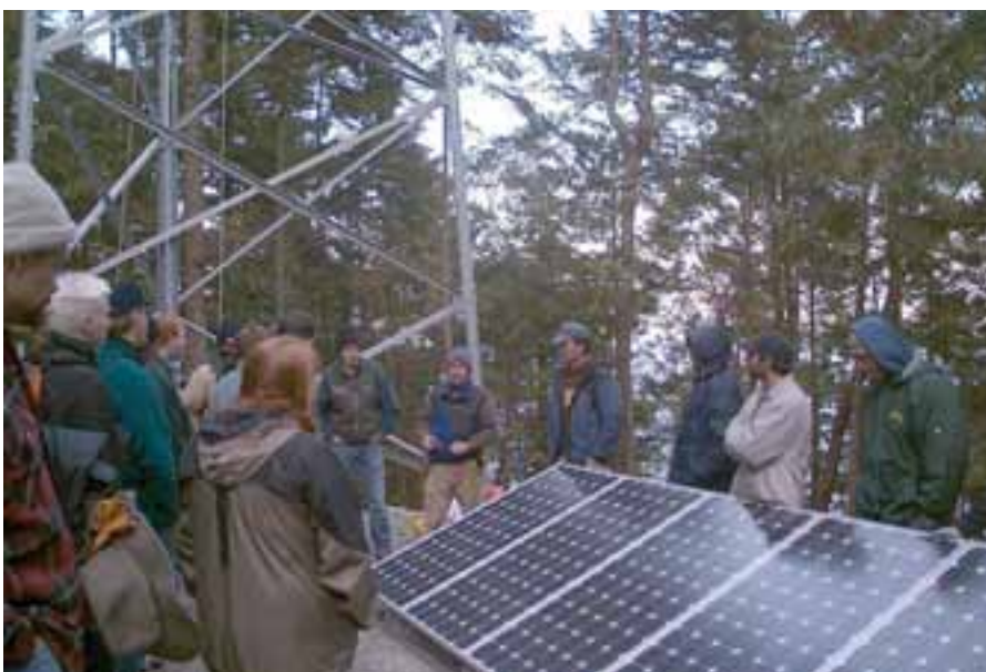
Kelly Keilwitz and E. H. Roy give SEI students instructions on the procedure for lifting the first array for placement on the tower.
