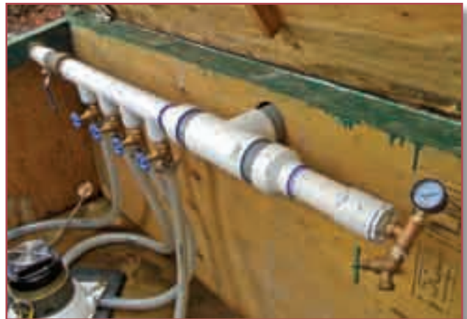
Four valves control flow to the four nozzles, while a pressure gauge monitors system head.
