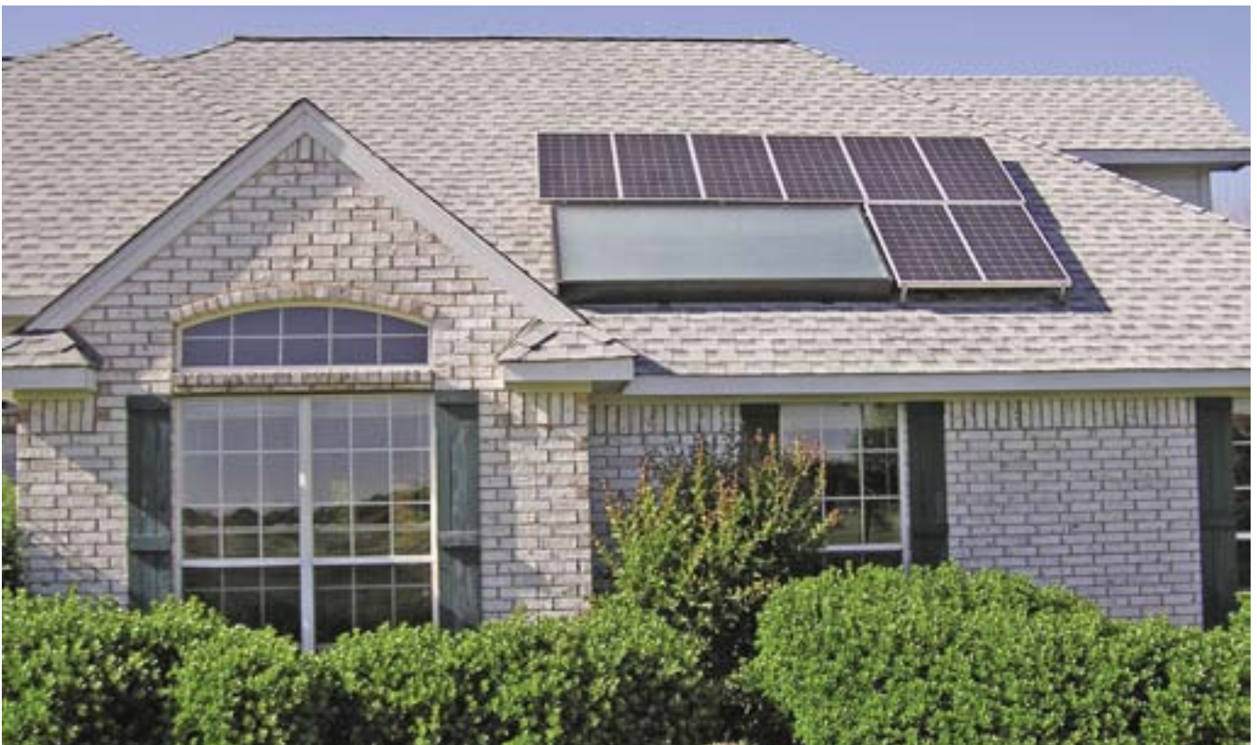
A batch water heater mounted on the garage roof (alongside the solar-electric array) meets a large portion of the Geisler family's hot water needs. The 880-watt, utility-intertied array offsets electrical use by about 15 percent.
