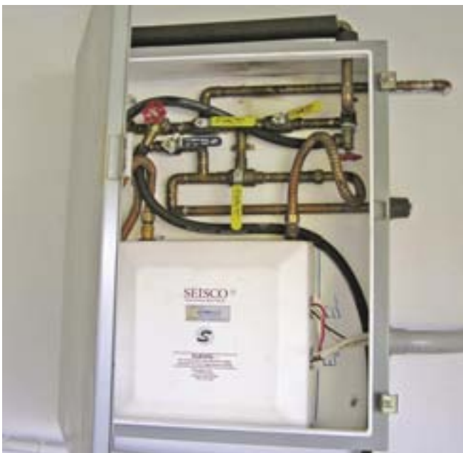
An energy saving, on-demand, tankless water heater serves as a good backup to a solar domestic hot water system.
