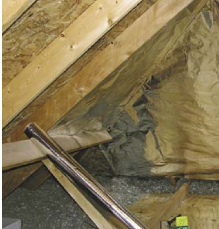
Installing a radiant barrier under attic rafters can considerably reduce heat gain through the roof.
